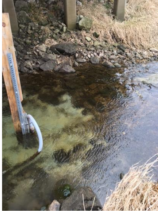
Figure 64. Streambed scouring and bare clay beneath the pressure transducer at Site 5 after Storm 17. Note the transition from the scoured pool section of the stream to the run with larger cobbles and boulders.
